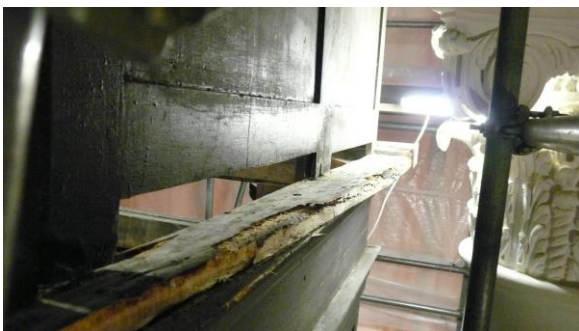
The Bass impost compromised by (historic) vermin attack
