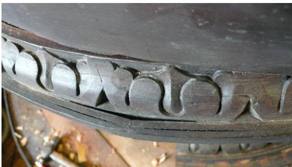
Laminated moulding coming apart because of shrinkage
