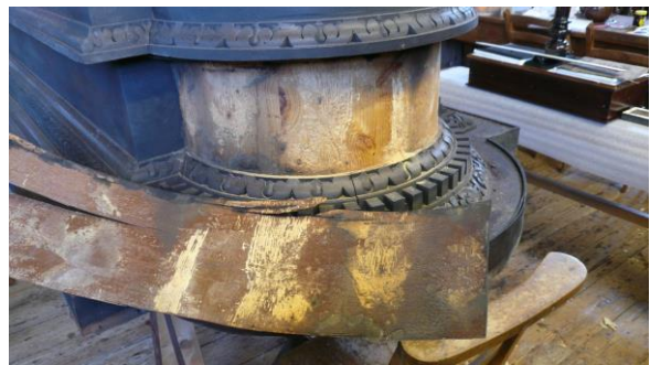
Woodworm damage to the pine sub-structure
