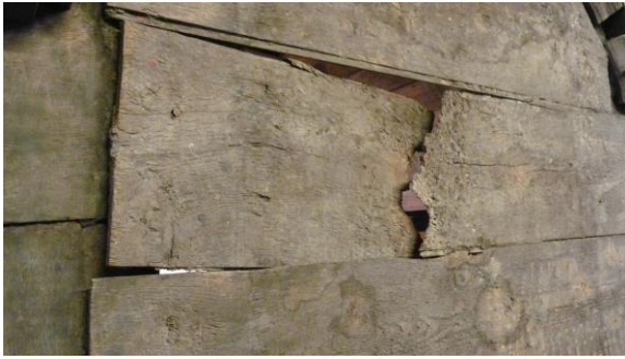
A broken roof plank
